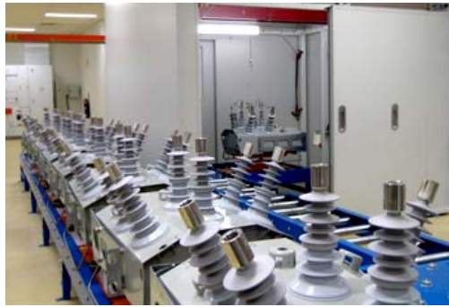
High Voltage Test Area
